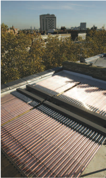
Solar water heating installation on the Flagship Home, London courtesy of the Royal Borough of Kensington and Chelsea
