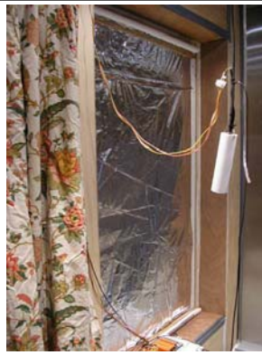
7. As Option 5, with low emissivity plastic film fixed to the room facing side of the blind U value 2.6 Heat loss reduced by 46%
